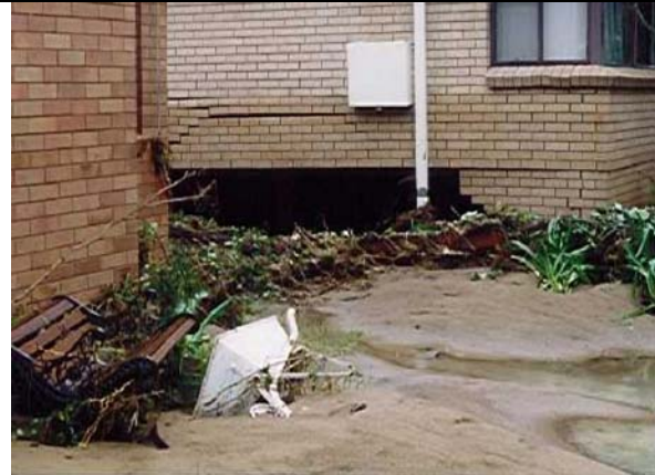
Fig. 30. Damage to brick building
